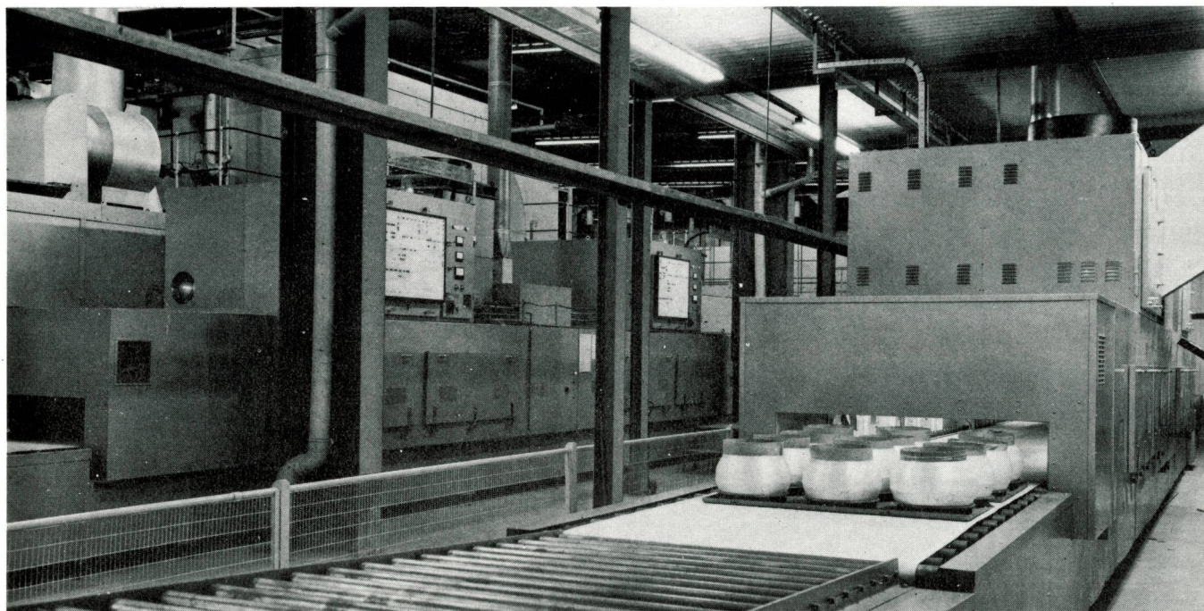
Feed end of cake drying unit. Another 50 x 50 kw series equipment can be seen in the background
